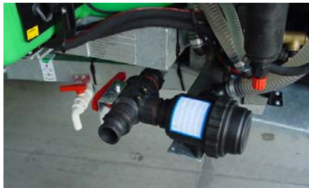
3-way deviator for filling tank
